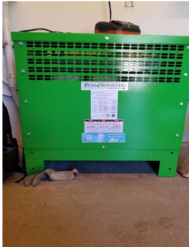
New energy efficient transformer
