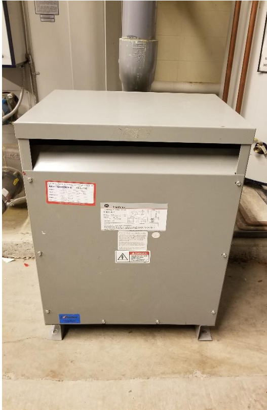
Older existing transformer
